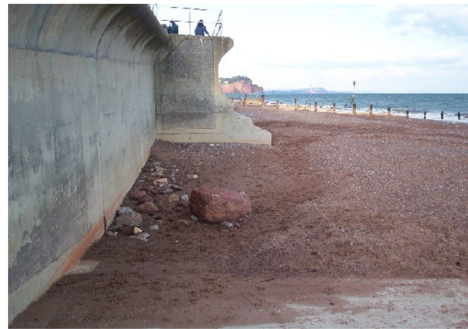
Left: An example of scour at a seawall in Teignmouth (southwest England) after a severe easterly storm, showing beach lowering near the base of the structure. Beach levels in this photograph are approximately 2m below 'typical' levels.
