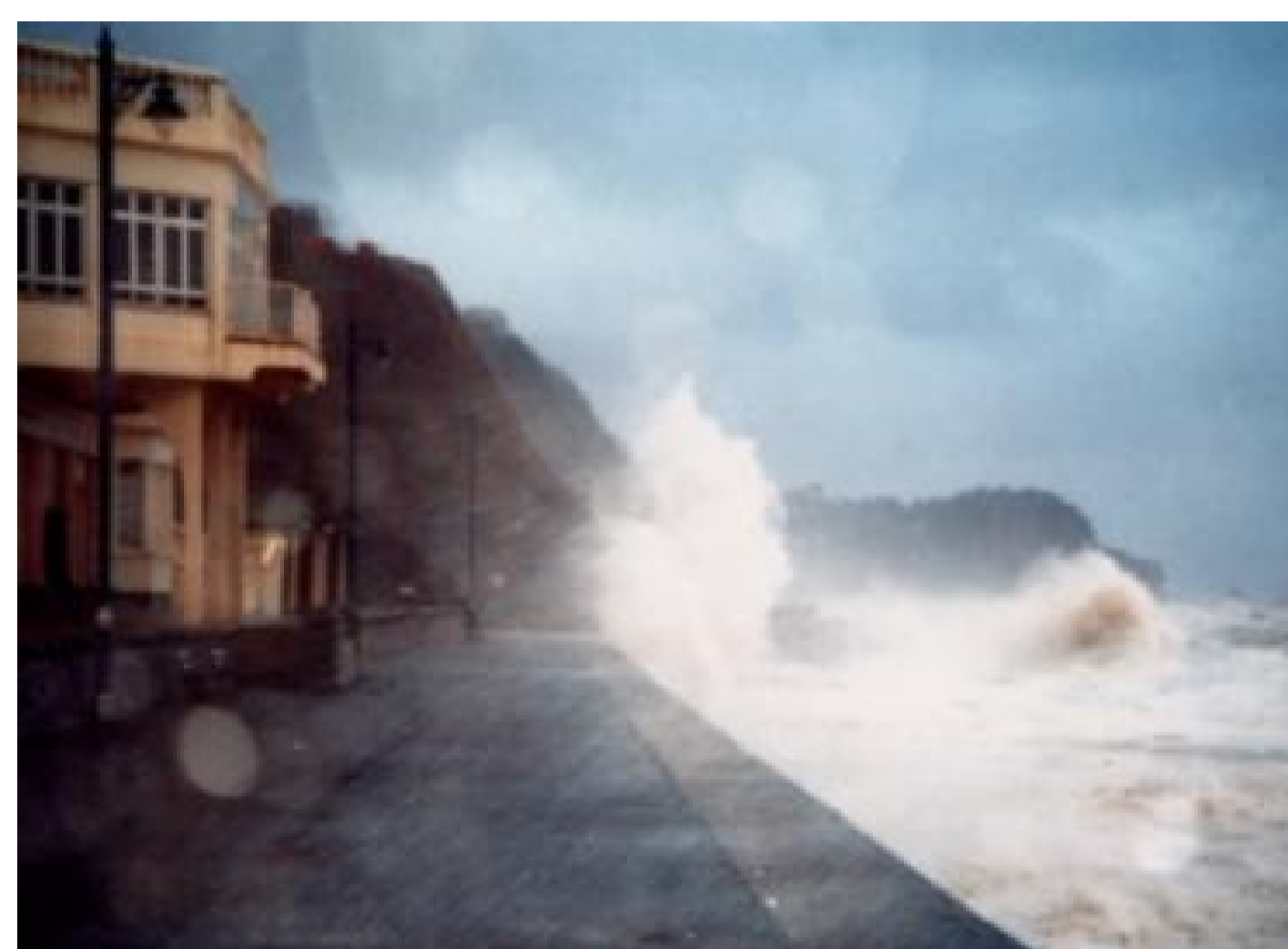
Above: Examples of wave overtopping. Overtopping resulted in the temporary closure of the London-Penzance mainline railway and extensive damage to sea defences along a large portion of the South and Southwest coastline of the UK.
