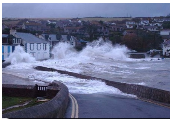
Figure 1: Wave overtopping of a seawall in southern England. The overtopping resulted in the temporary closure of a mainline railway and extensive damage to sea defences along a large portion of the south coast.
